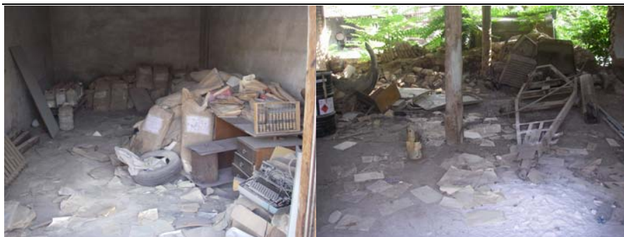
Figure 4.10 Overview of the room with big quantity of DDT and of the shed the wall at the back is completely gone
